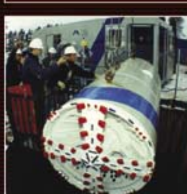
Bottom: Superintendent Bob Welch and crew start slurry micro-tunneling using Ackerman MTBM. New Hampshire.
