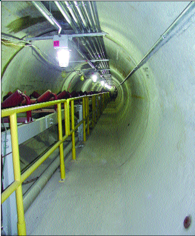
Bradshaw Construction recently completed a unique project in Washington, D.C., for coal conveyance using pipe jacking to install 96-in. RCP
