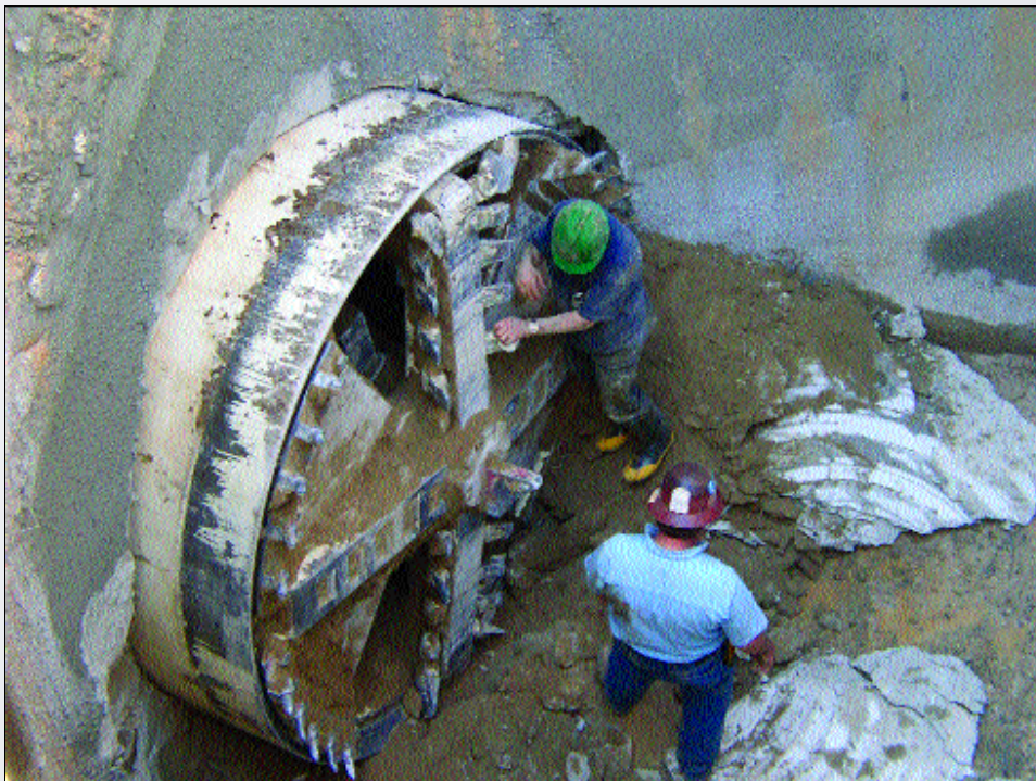
A 101-in. Lovat TBM holes through on a project Bradshaw Construction completed on the University of Virginia campus in Charlottesville.
