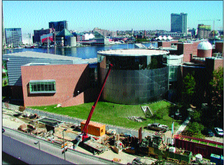
Building underground facilities increasingly requires working in proximity to existing utilities and structures, like this project in Baltimore's Inner Harbor.
